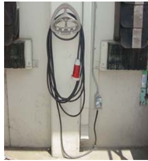
Shore Power: 208 Volt, Single Phase
